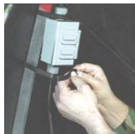
Don't overload receptacles.
